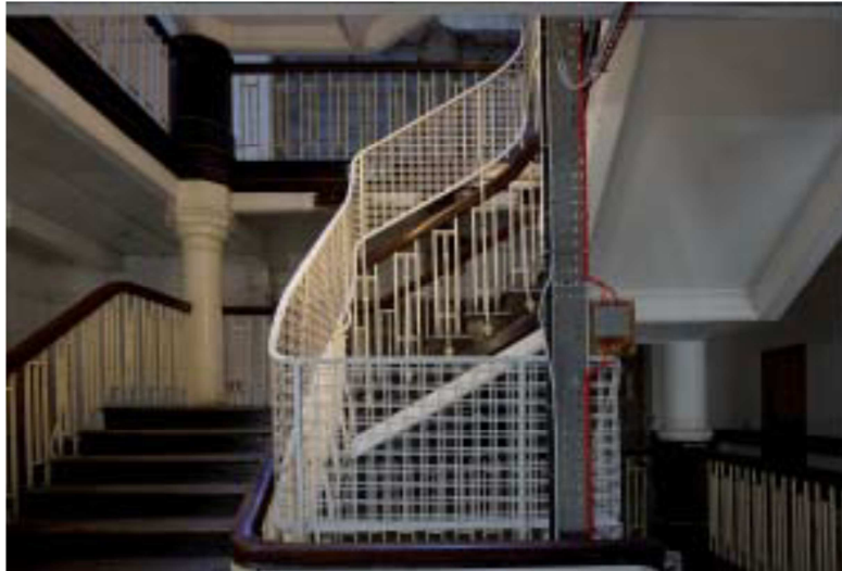
Image showing stairs located within eastern part of the building including steel framed balustrade with timber handrail. A similar staircase is located within the western part of the building
